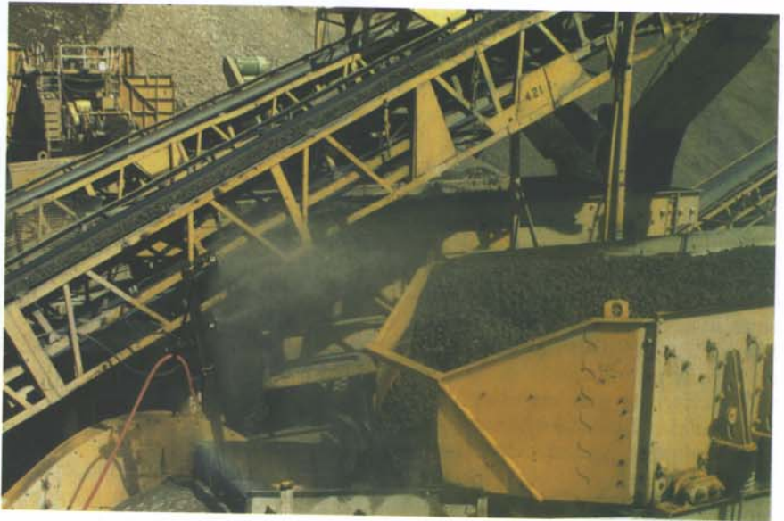
An Arch simplicity impact system and at-last-a-sealing system installed at a conveyor transfer point.
