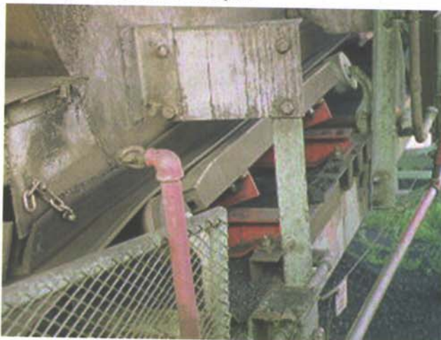
An Arch fogger system suppressing dust over an open discharge chute of a conveyor.
